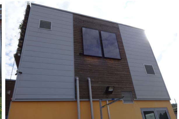
Concrete and wood facade with thermal solar panel.
