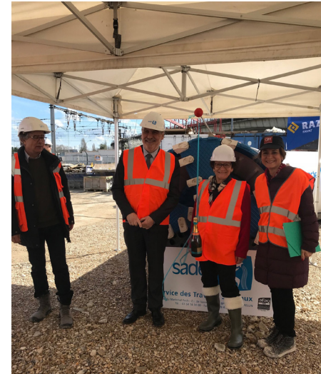
In presence of Mr. Christian FAVIER, President of the city department of Val-de-marne, M. LOBADA, DSEA 94, and Josiane MARTIN, godmother of the microtunneling.
