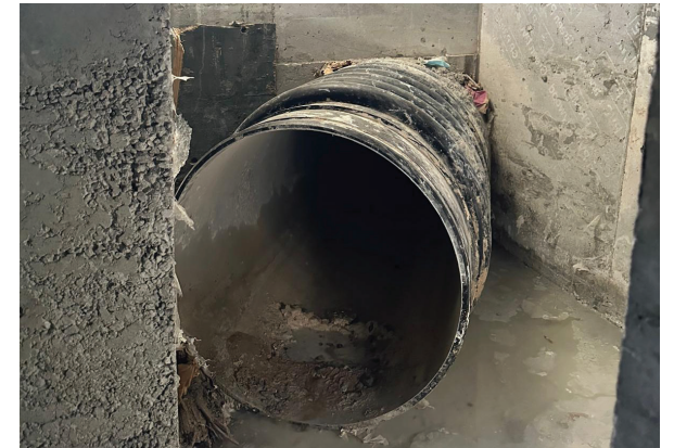
Air outlet of the Canadian well inside the building, LGF
